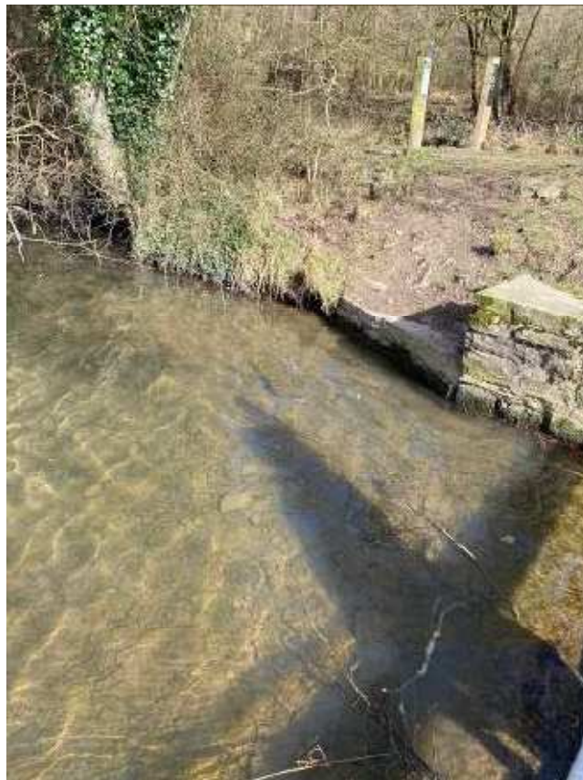
Undermining – upstream left side
